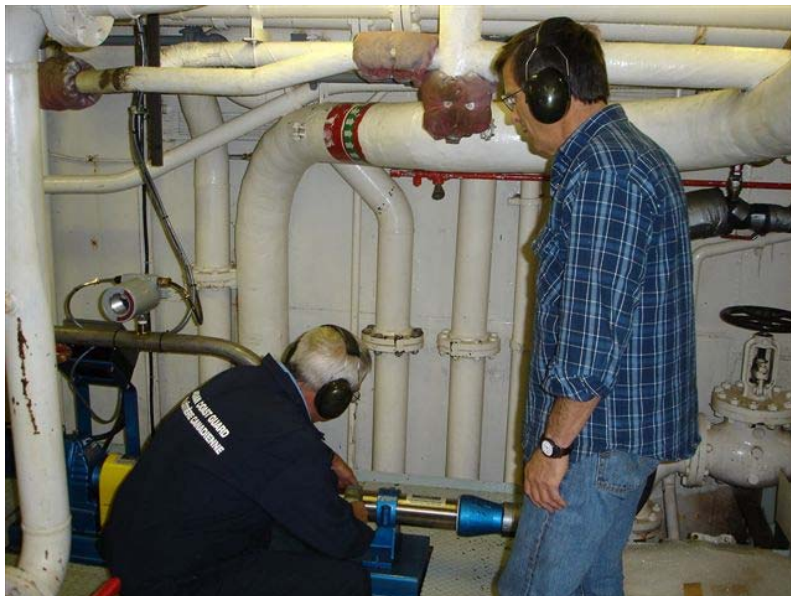
Figure 2. Pump for seawater loop at intake in engine room (2007 photo)
